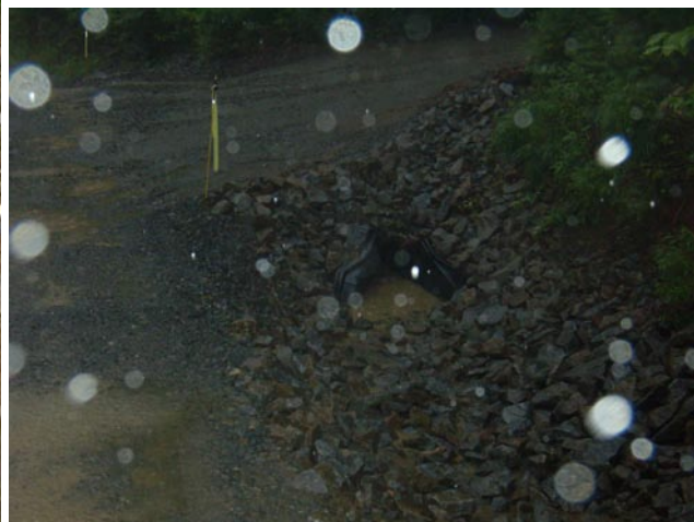
Photographs of culvert under Jackson driveway taken on June 30, 2009. Photo on left was at the beginning of a rain event. Photo on right was taken 20 minutes into rain event. Notice the increase in sediment laden runoff at the entrance to culvert. Photo directly above is of culvert discharge during rain event.
