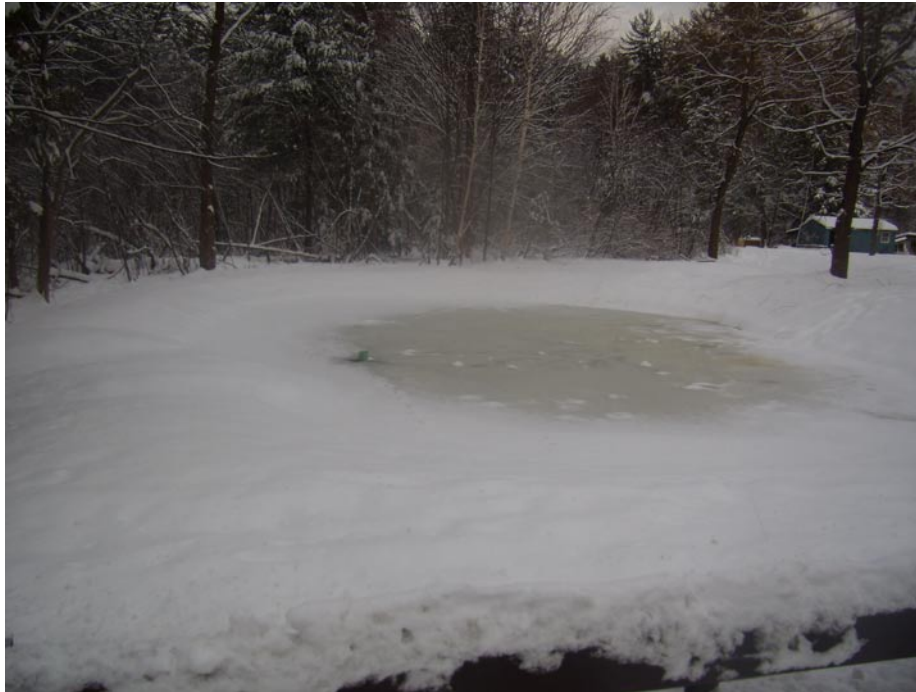
Photograph of wet pond constructed at the Blue Lagoon Resort. Note the standpipe on the left side of the pond and the ice elevation which reduces the ability for stormwater management.
